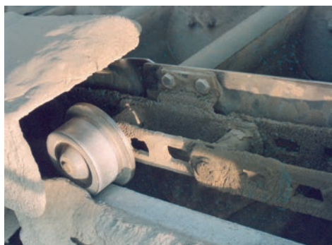
Bucket apron conveyor for clinker.
